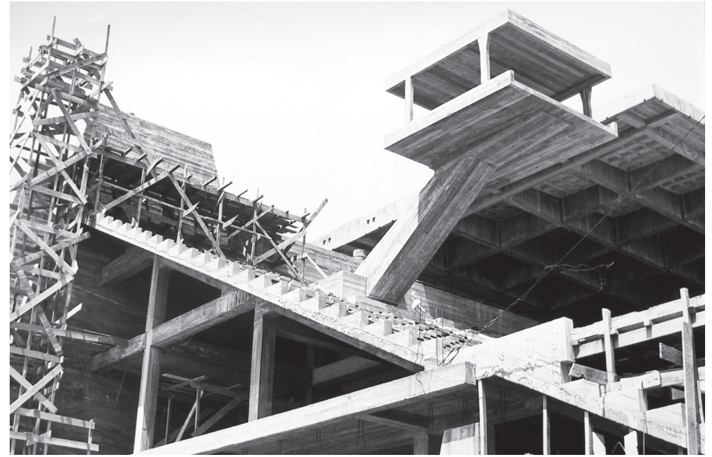
The National Sports Complex (Olympic Stadium), Phnom Penh under construction, 1963. Collection Vann Molyvann
